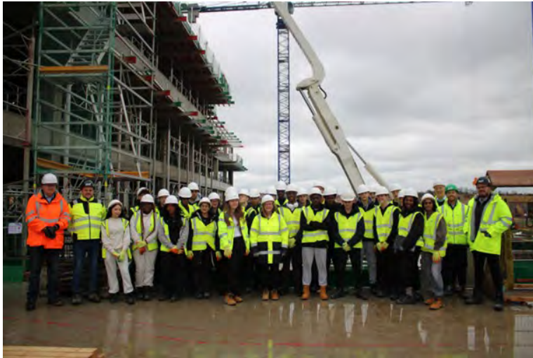
Image taken on site of the Alkerden Academy where students attending the Building Future Skills Programme in Ebbsfleet were given hand-on experience of life on-site.
